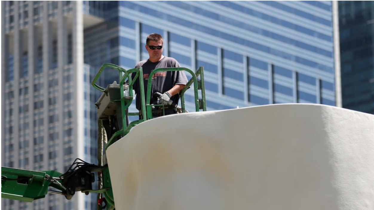
Ironworker Mike Grecnik works with a crew to erect a 39-foot high sculpture "Looking Into My Dreams, Awilda" by Jaume Plensa, the renowned artist who also designed Millennium Park's Crown Fountain.
