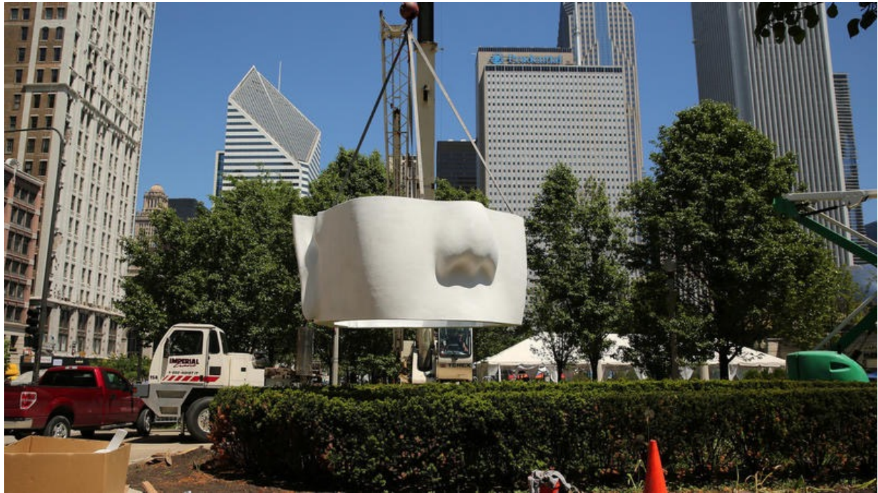
A section of sculpture hangs suspended from a crane as a crew works to erect a 39-foot high sculpture "Looking Into My Dreams, Awilda" by Jaume Plensa, the renowned artist who also designed Millennium Park's Crown Fountain.
